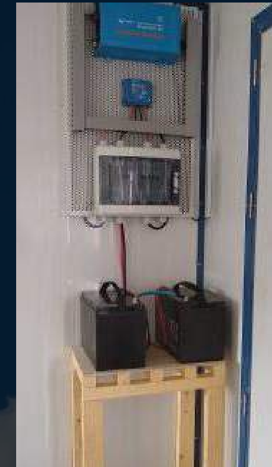
Solar panel control
